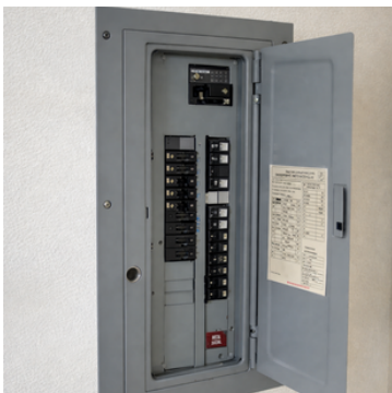
Electrical panel - compliant
