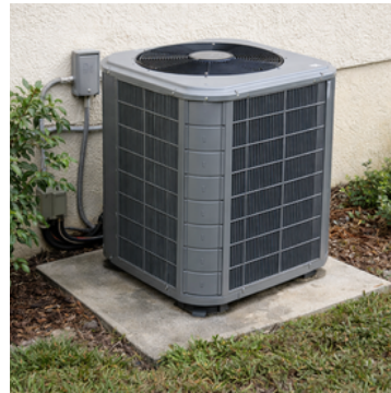
HVAC unit - operating normally
